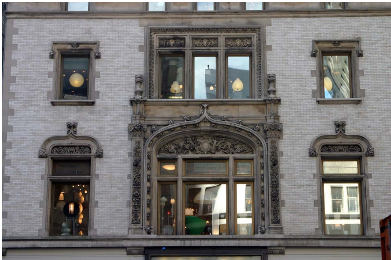
Society House of the American Society of Civil Engineers Fourth Story, Cornice and Parapet (upper); Second and Third Stories (lower)
