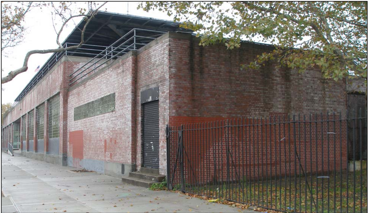
Betsy Head Play Center Men's shower room and stairs to roof deck (now enclosed) Photo: Christopher D. Brazee, 2007
