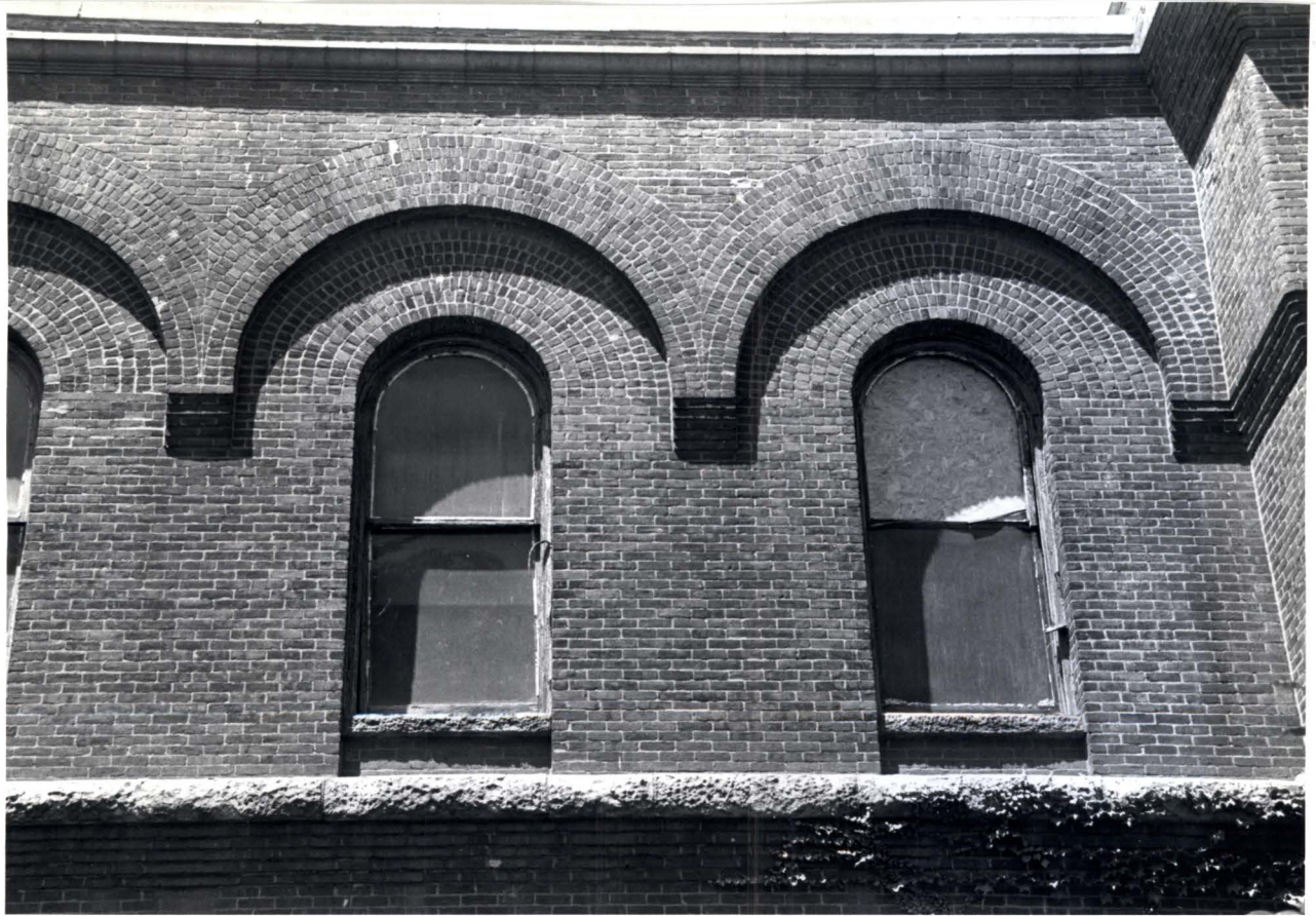
14th Regiment Armory, 1402 Eighth Avenue, Borough of Brooklyn. Window detail, Administration Building. Photo: Carl Forster, 1997.
