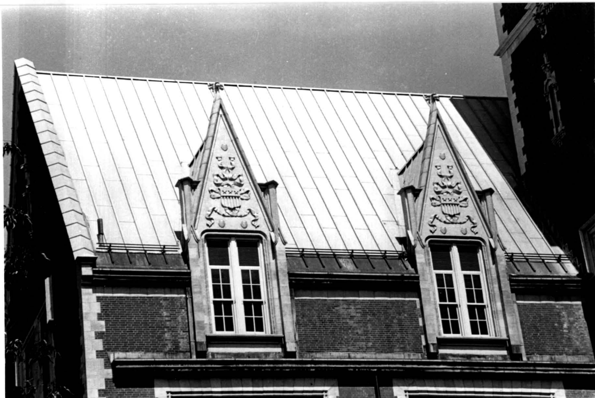
Fig. 6: Wadleigh High School for Girls (1901-02). Detail of dormers. Photo Credit: Carl Forster.
