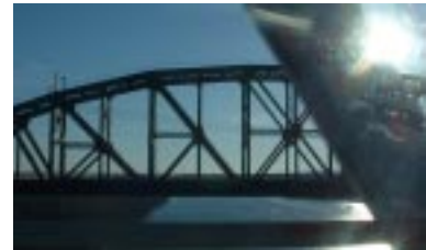
Figure 4.26: Many bridges are essentially trusses. Here's one that is partially obscured by the truss on a car bridge.
