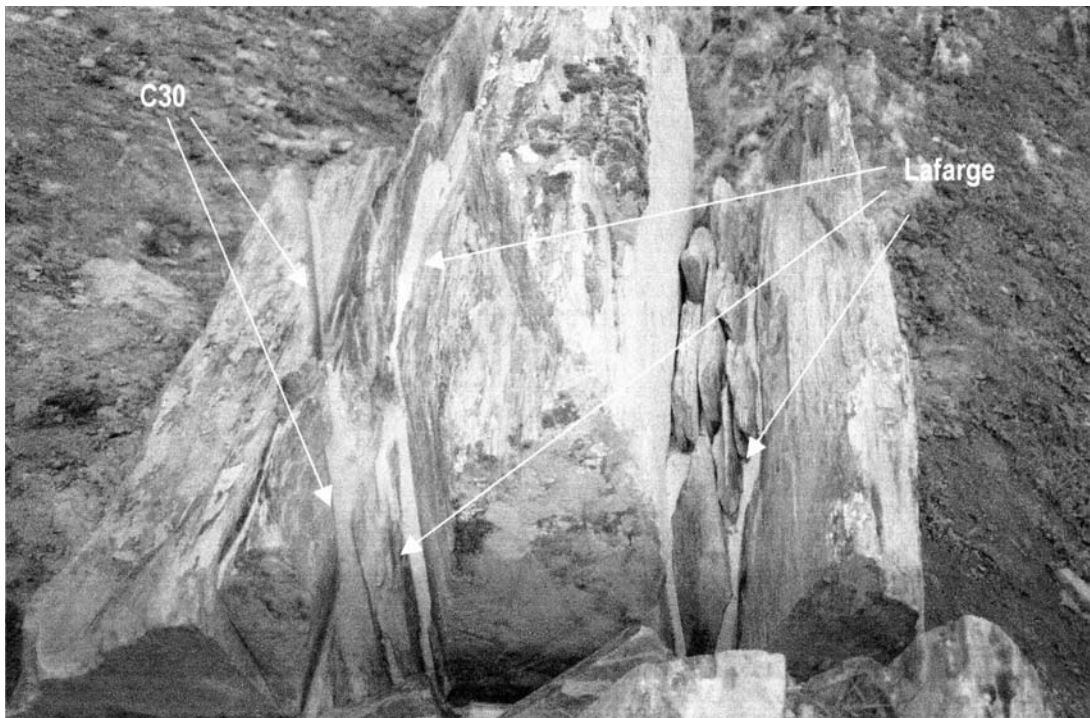
Figure 10.8. Penascosa Type-Rock after In Situ's treatment with indication of the zones where two distinct mortars were applied. (Photo: In Situ).
