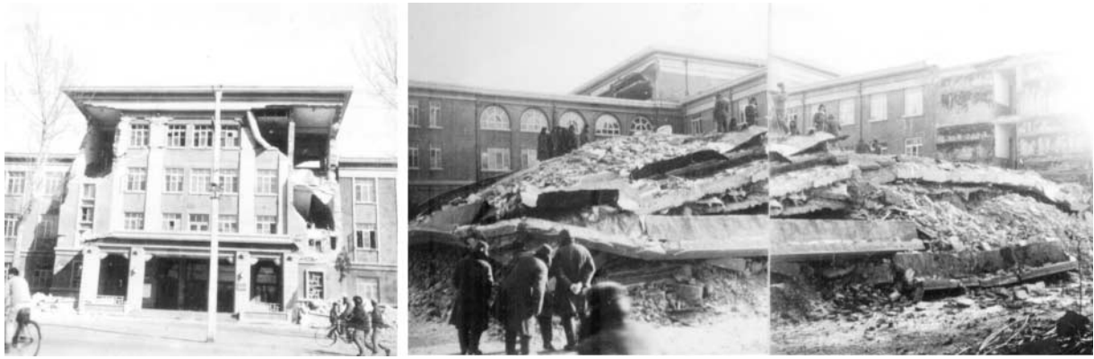
Figure 8. Damaged building of the Haicheng guesthouse (built with bricks and concrete). The building had an E shape in plan view, with the three back wings oriented perpendicular to the front wing. Left: Front view. Right: Back view, two side wings at the back collapsed. The center back wing did not collapse (shown in the background on the left-hand side).
