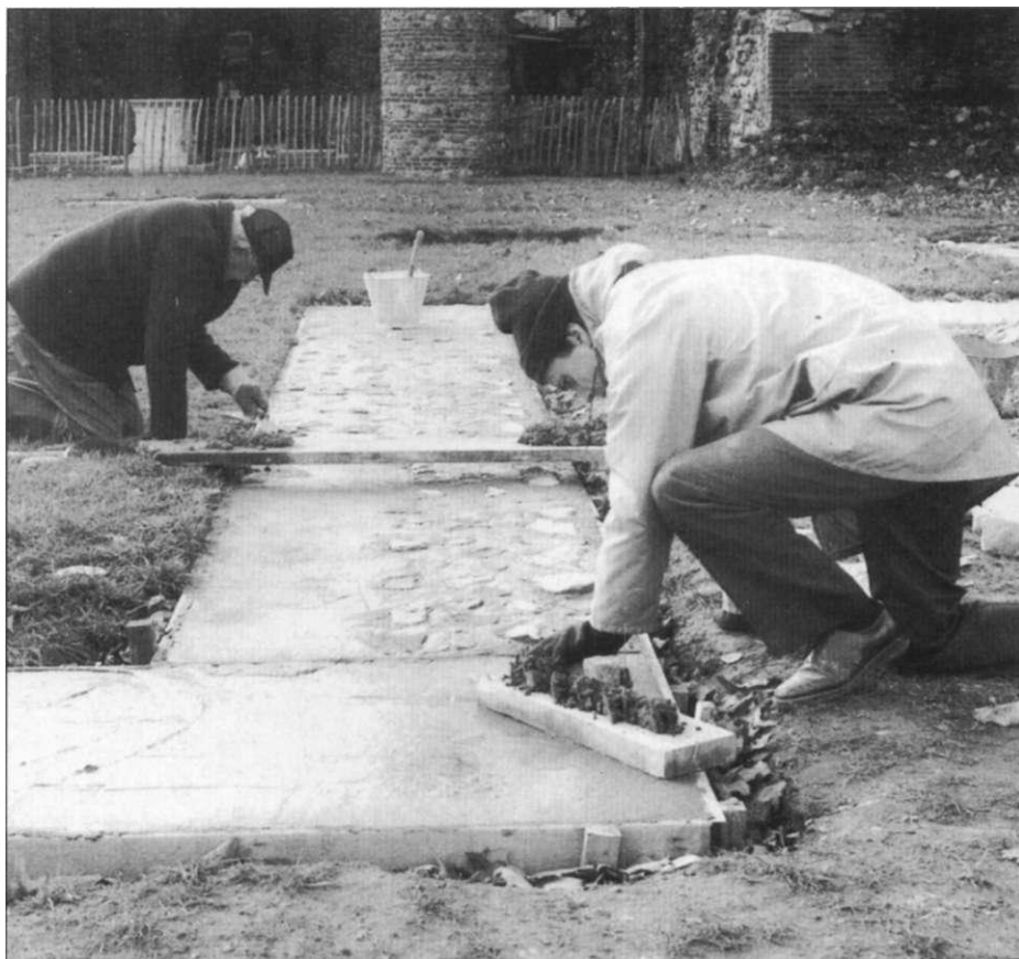
Dennis Tripp and Donald Shimmin temporarily join the building trade at St Botolph's Priory.
