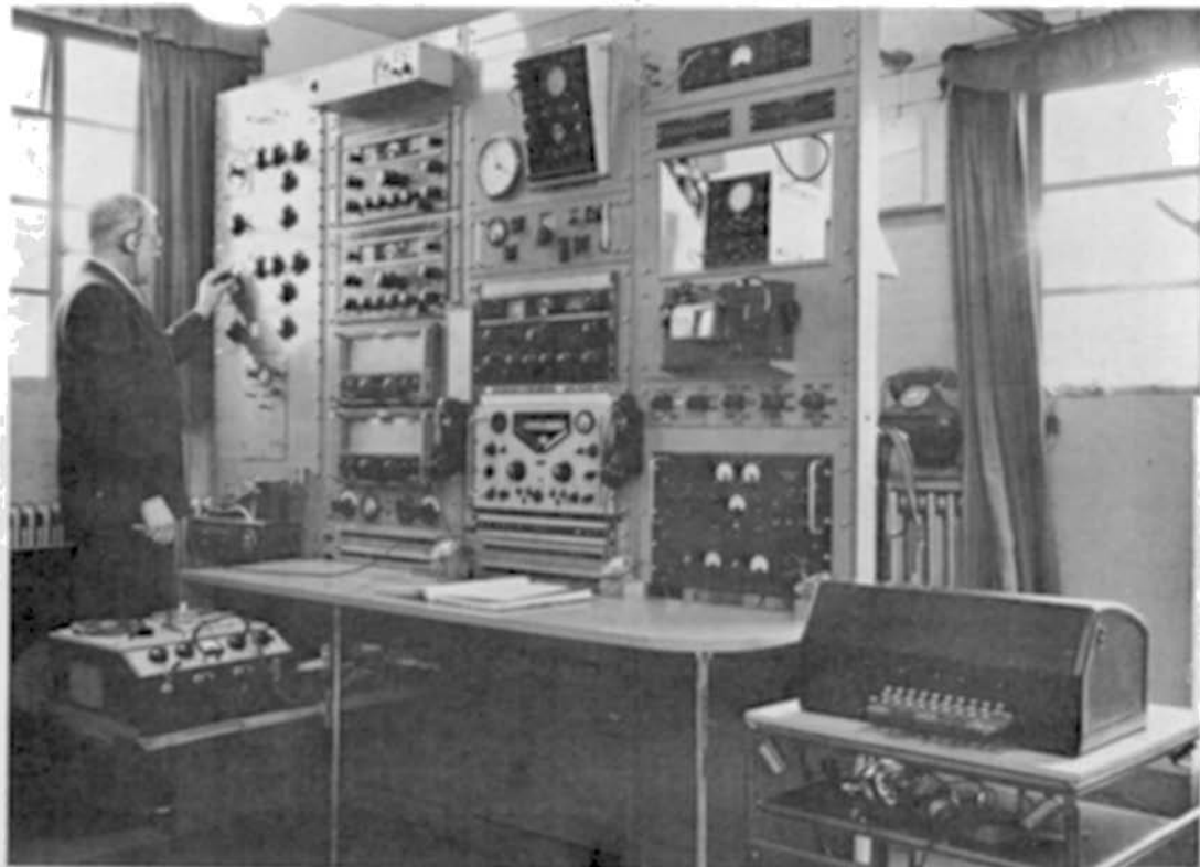
Equipment bays in the Operational Supervisory Room (S.M.E.s' Room): On the right is the teleprinter receiver.
